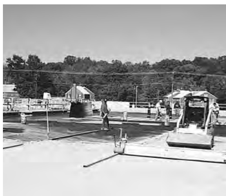
Figure 18. A mechanical screed used to level bedding sand on a roof parking deck project.
