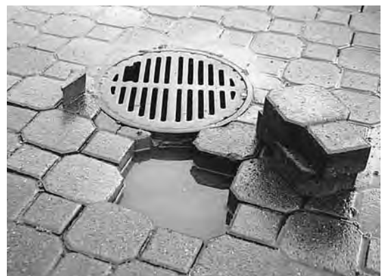
Figure 15. An absence of holes in the sides of this roof drain led to ponding.
